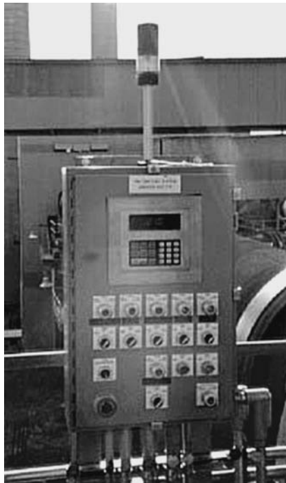
FIGURE 1.9 Tire fuel control panel with weight indicator at the cement plant.
